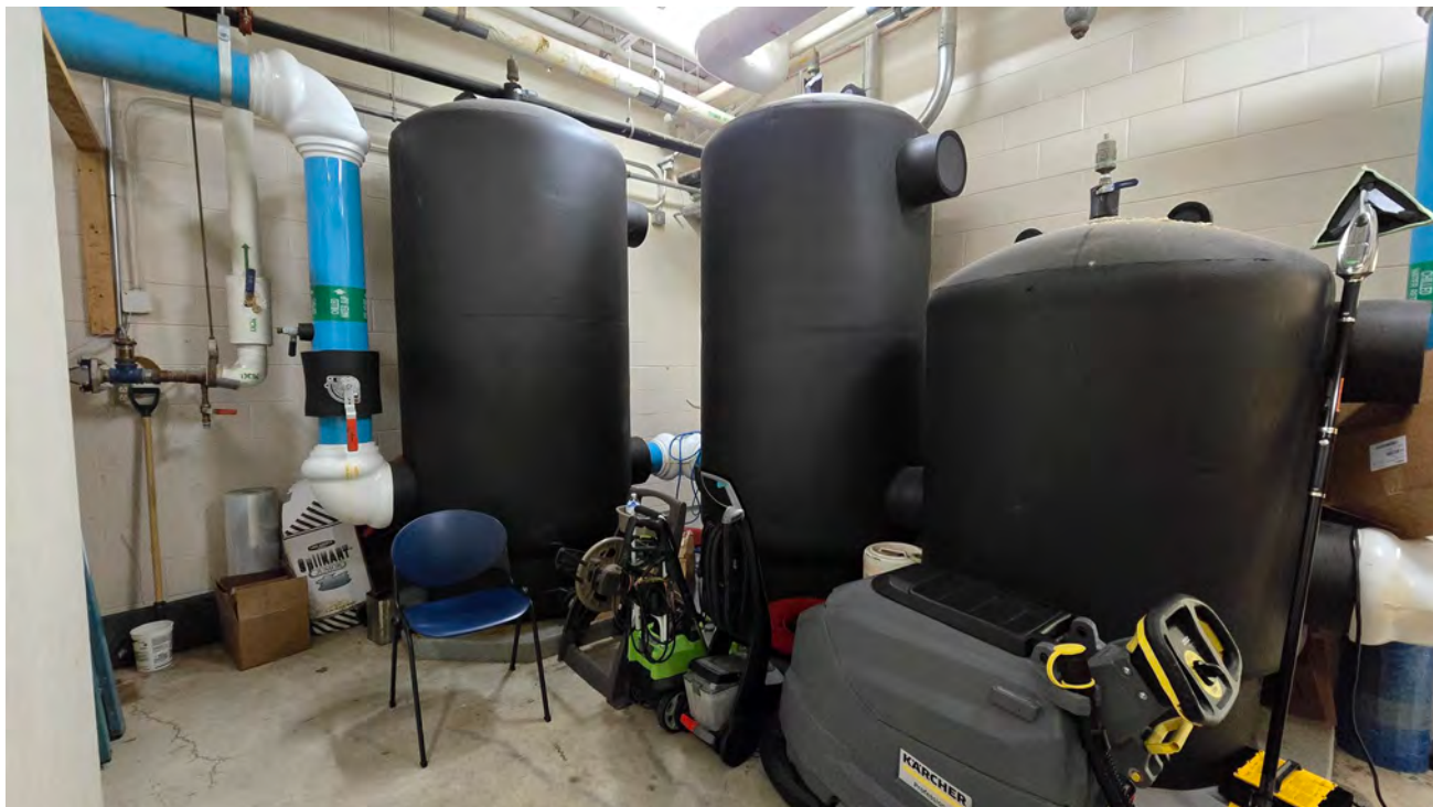
Photograph # 17: Water supply system in first floor equipment room.
