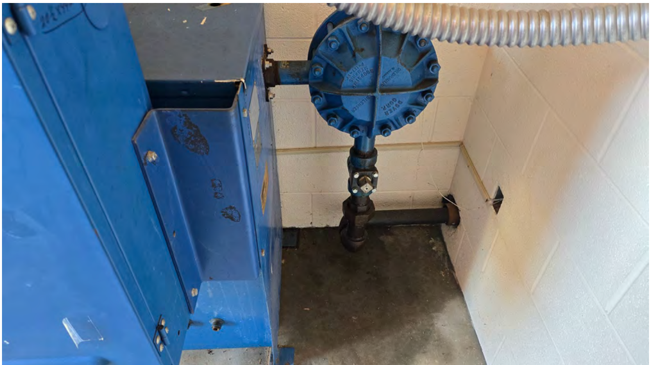
Photograph # 16: De minimis oil staining near elevator hydraulic equipment.
