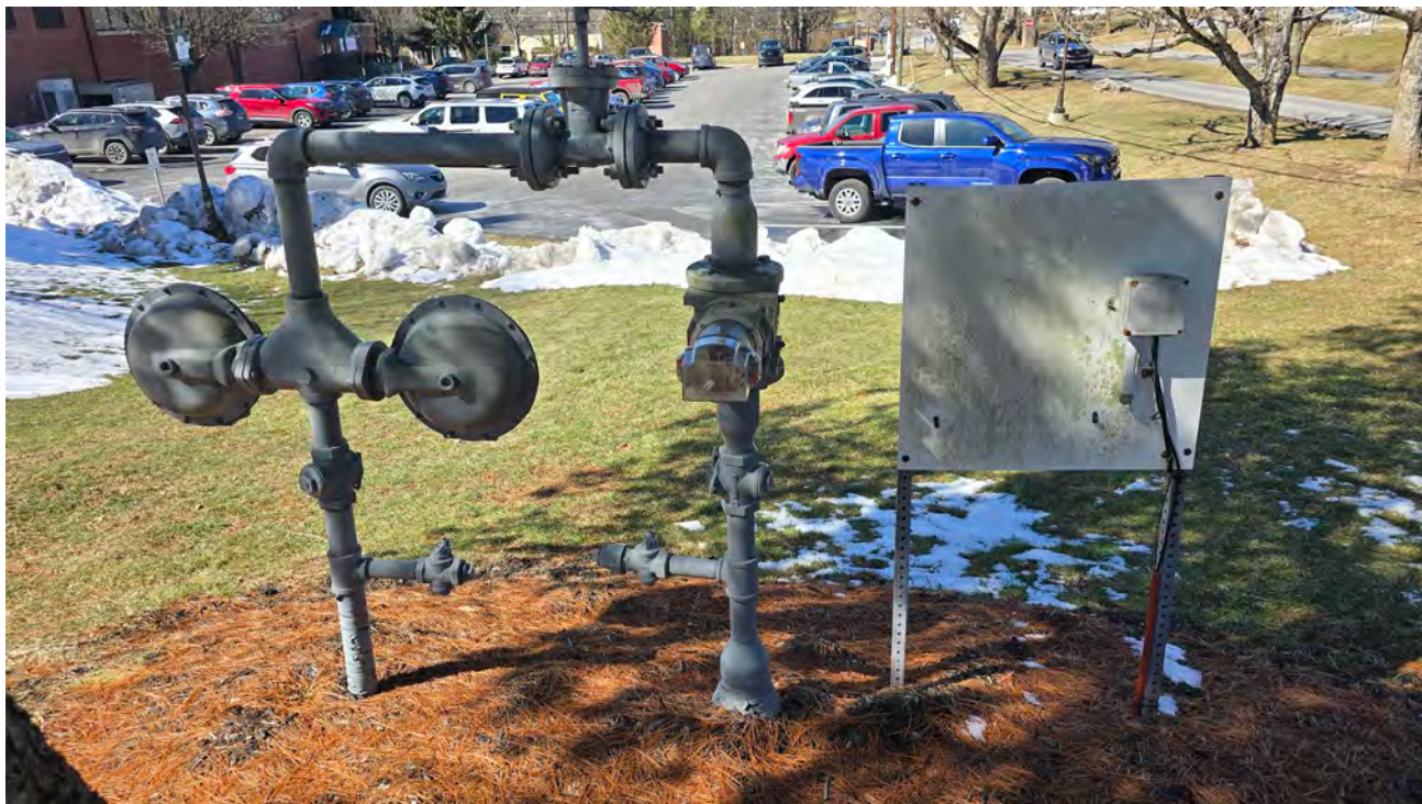
Photograph # 3 WVSOM gas meter located on the northern corner of site.
