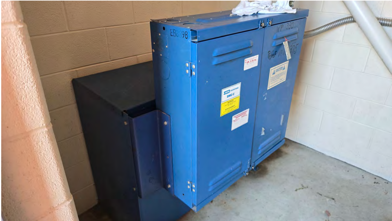
Photograph # 15: Elevator hydraulic equipment room on southern building face (exterior entrance).
