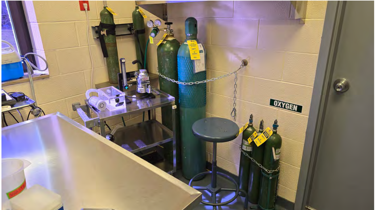
Photograph # 23: Gas cylinder storage in surgery suite.
