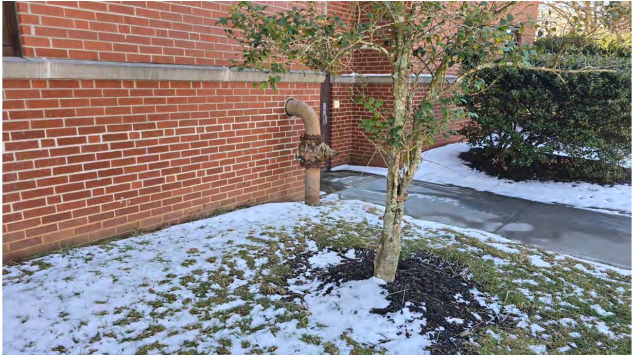
Photograph # 11: Water service line entering building on western building face.
